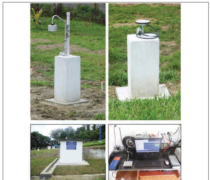
Figure 33 AEFM and GNSS receiver field installation at MO, Silchar
